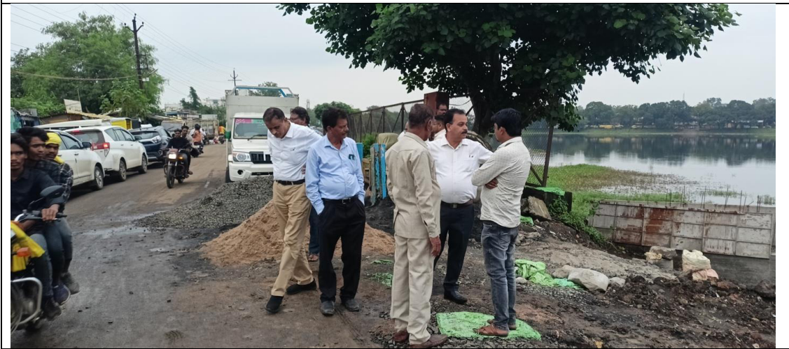
Damaged Lake bund, fencing and pathway
